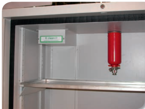
Fire-extinguisher installed in a safety cabinet
